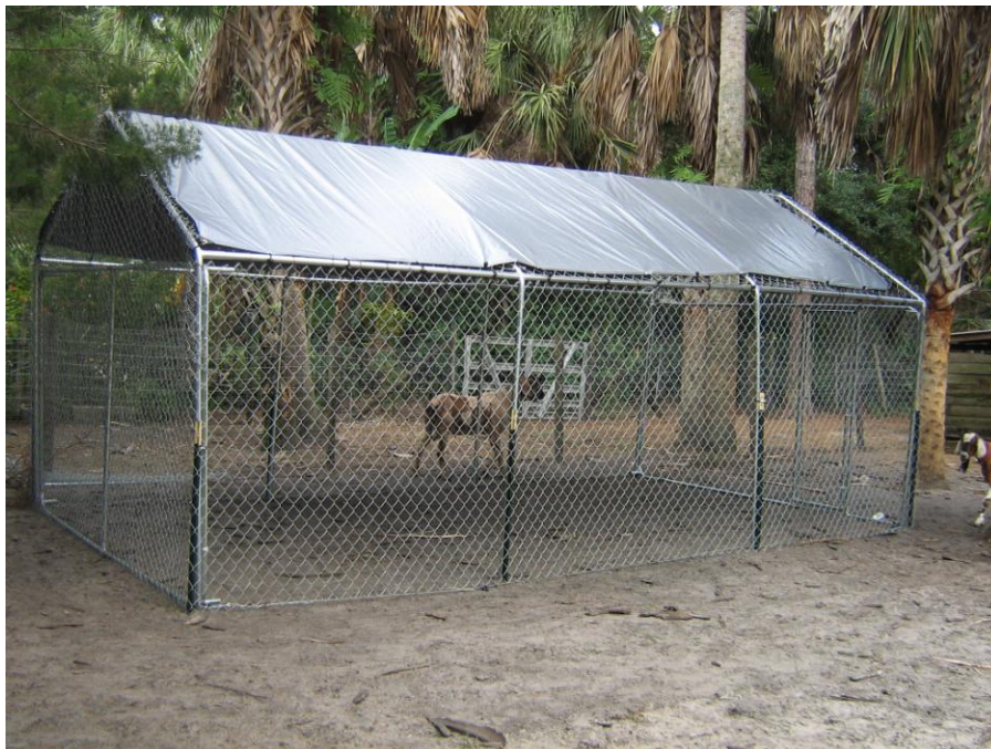
Construction of a proper livestock enclosure is the only sure fire way to protect ones animals for those living in panther country.
